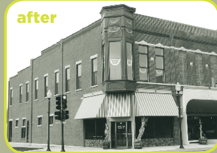
A new awning, tuck pointing, and new upper-floor windows turned this declining asset into a shining asset in Charles City, Iowa.
